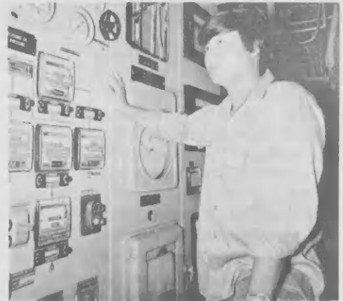
Clifton Ahlip, mechanical student, becomes acquainted with recording instruments at Powerhouse No. 1.
